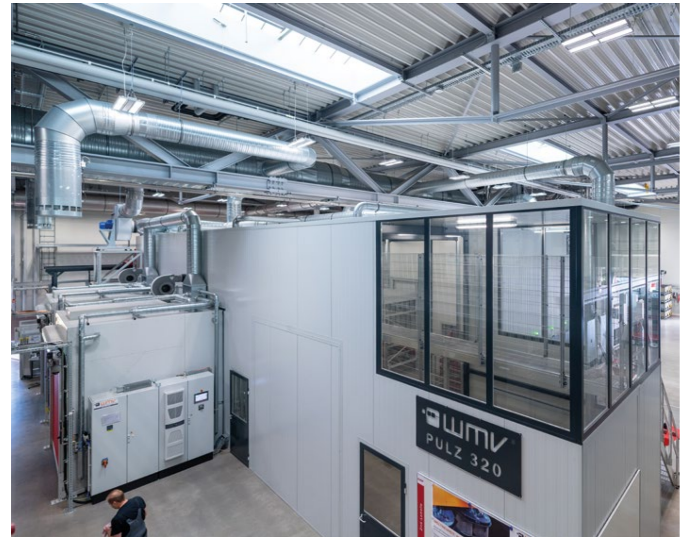
Modern plant technology for zinc-flake coating at the EJOT site in Tambach-Dietharz
